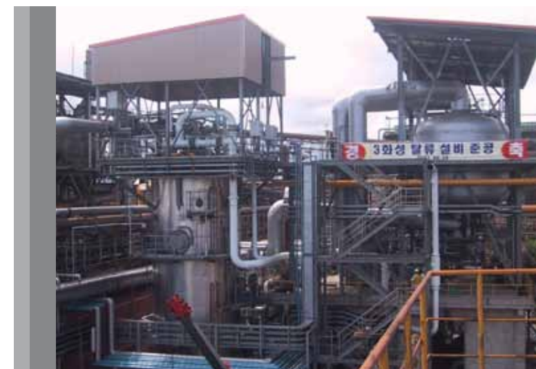
Claus Plant for Sulphur Production
