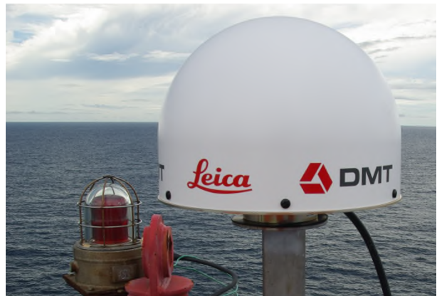
GNSS Choke Ring Antenna, mounted on a platform.
