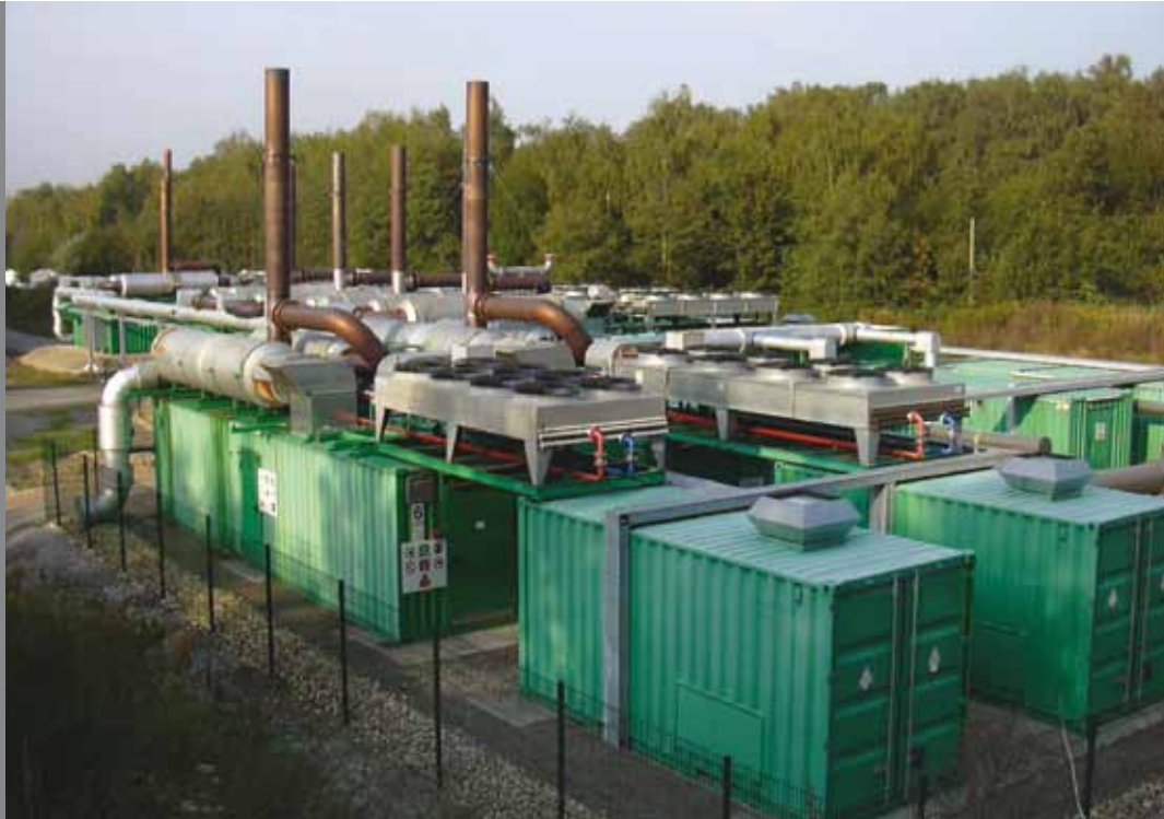
Containerised CHP-plant (courtesy of Minegas GmbH)
